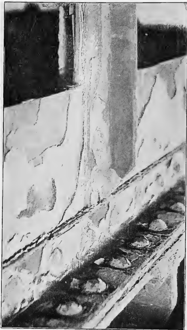
Rust on a neglected highway bridge
